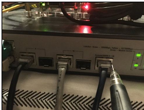
Switch Ethernet cable
