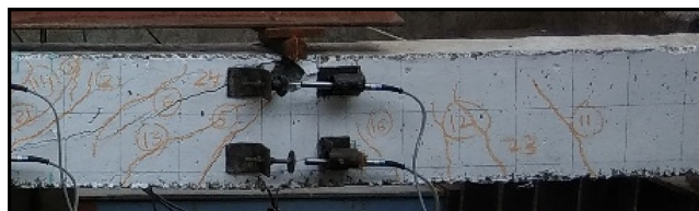
Figure 17. Crack pattern at the center of the span for the M_{100} grade HPC 100DB2 beam specimen. Photograph courtesy of Aijaz Ahmad Zende. Copyright 2023.
